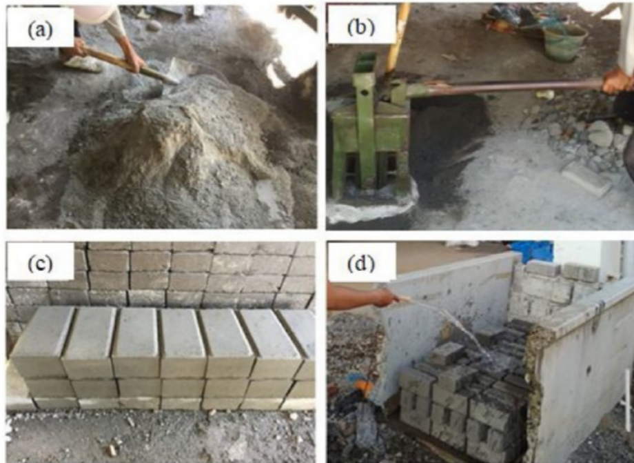
Fig. 5. Procedure for making the paving block (a) mixing; (b) compacting; (c) fresh blocks; (d) curing method.
